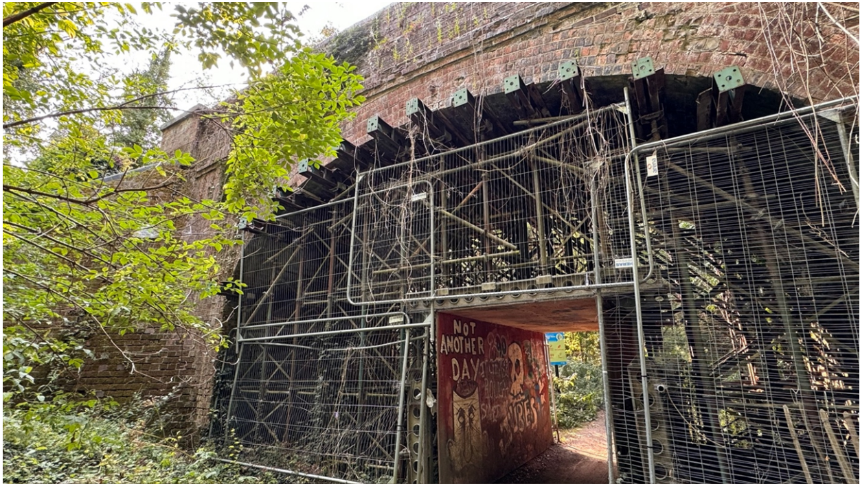
Bridge view towards Haverhill, showing condition and existing propping
